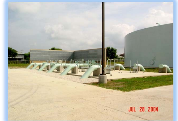
Micron Pump Station, 2003
