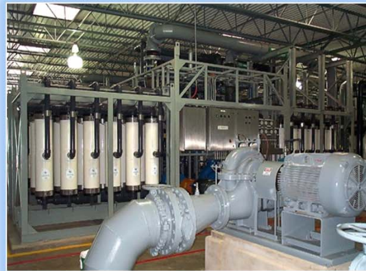
Medina River Plant, 2012 Ultrafiltration (Built by UWS in 1999)
