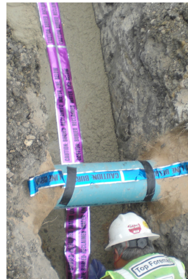
Figure 10.5 Purple warning label indicating reclaimed water pipe buried below
