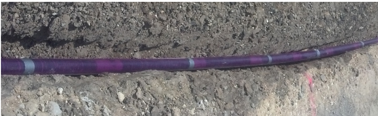
Figure 10.4 Color-coded purple label run lengthwise along top of pipe and taped firmly to pipe at regular intervals
