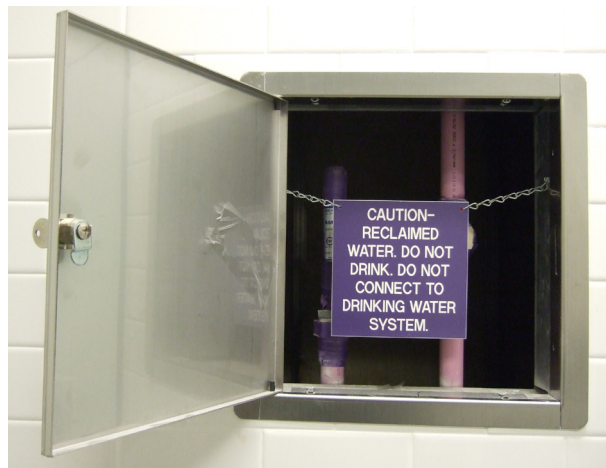
Figure 9.16 Appurtenance access in building wall with door open and proper signage
