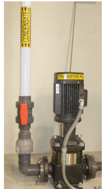
Figure 10.6 Condensate drainage pipe between AHU and storage tank
